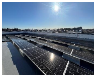
Photovoltaic Power Generation System
